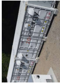
Conteneur de stockage batteries (source: ZE Energy)
