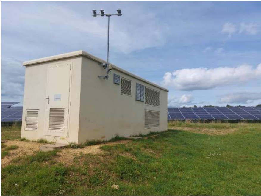
Figure 15: Poste (source TSE)
