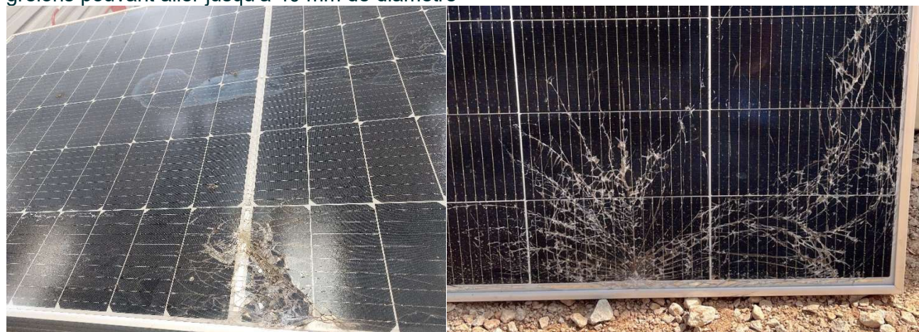
Figure 15: Panneaux ayant subi un impact (source TSE)
