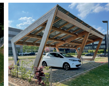
Ombrière photovoltaïque Source : www.service-aux-entreprises.com
