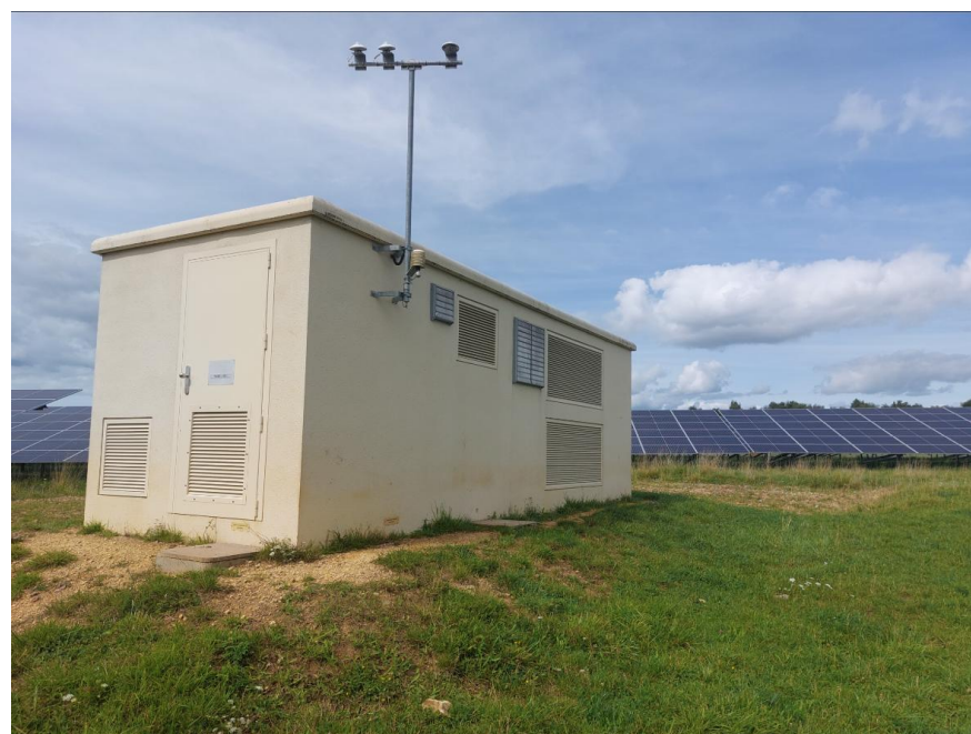
Figure 10: Poste (source TSE)
