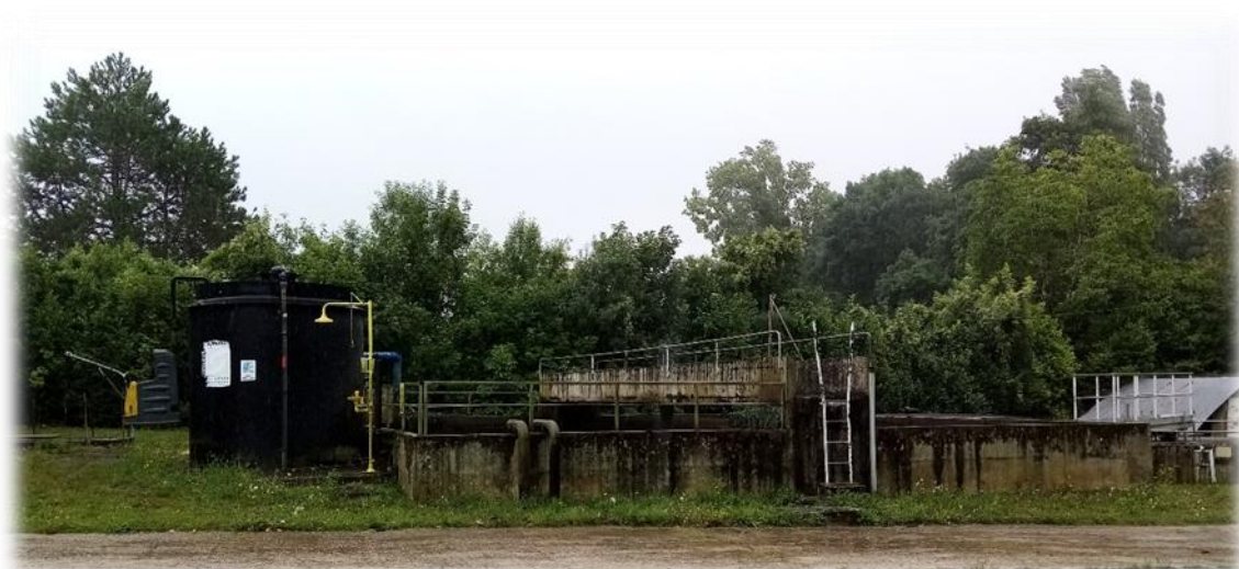
Figure 3: Station de traitement de Preuilley-sur-Claise
