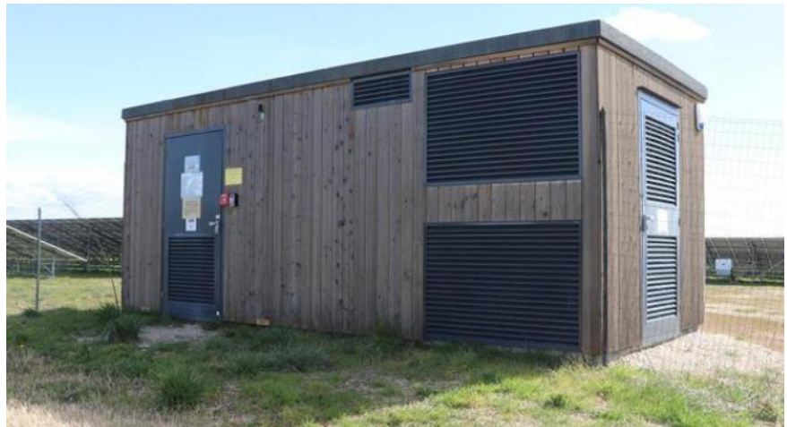
Figure 22: Exemple de local technique (source TSE)
