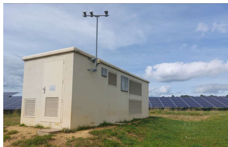
Figure 20: Exemple de local technique (source TSE)
