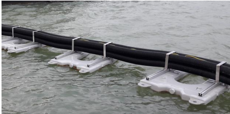
Figure 9 : câbles flottants partant des îlots (source : UNITE)
