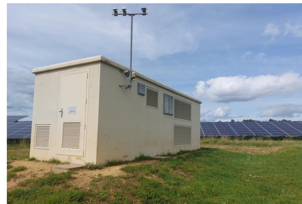
Figure 16: Exemple de local technique (source TSE)
